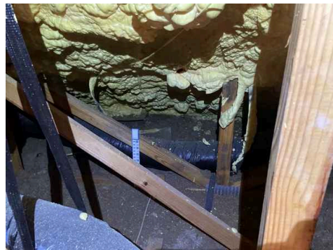
Blown insulation not removed prior to applying spray foam insulation
