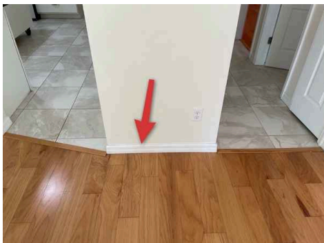
Baseboard separated from Front wall at rear of left hall closet
