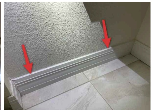
Baseboard separated from rear wall in left hall closet
