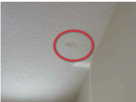
Stain on ceiling at rear right corner of living room
