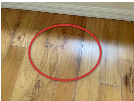
Possible water damage on floor below front dining room window
