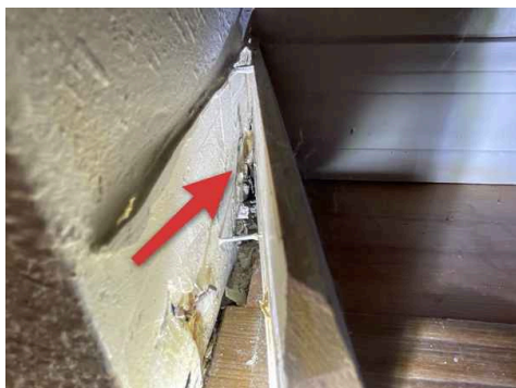
Behind baseboard at rear right side of front left bedroom closet, closet shares wall with air handler
