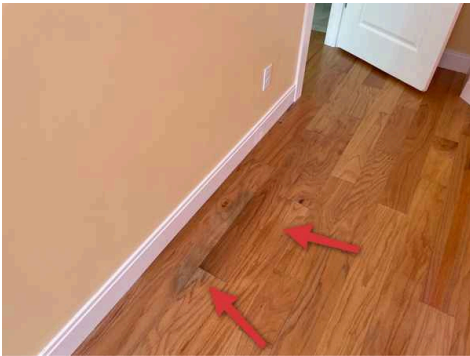
Possible water damage on flooring at right side of rear left bedroom
