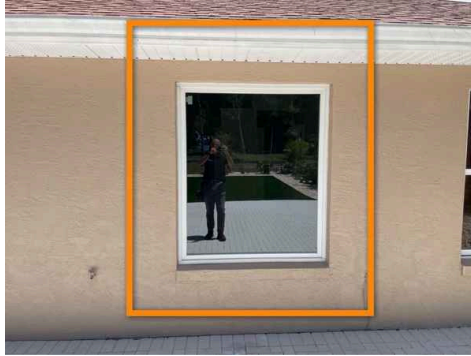
Multiple holes around window at rear left side of living room
