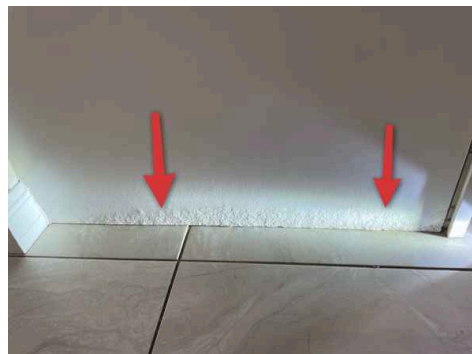
Water damage on end of kitchen cabinet, next to dishwasher
