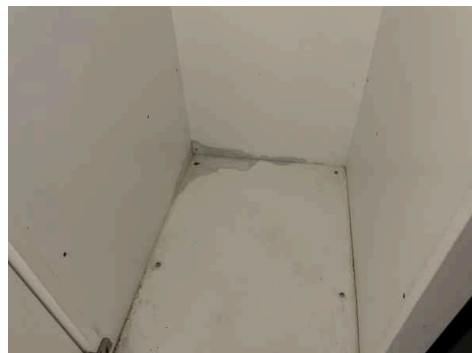
Stain inside laundry cabinet
