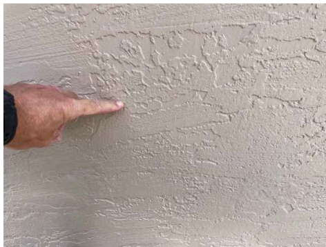
Left side by AC condenser
