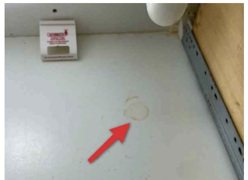
Stain on shelf below sink at right side of master bath
