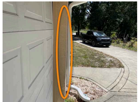
Multiple locations around overhead garage door
