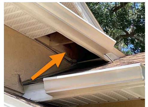
Missing it front right side
