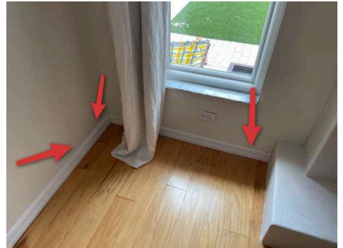
Baseboard separated from wall at rear left corner of living room
