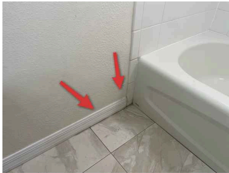
Baseboard separated from wall outside of left hall bath shower, across from toilet
