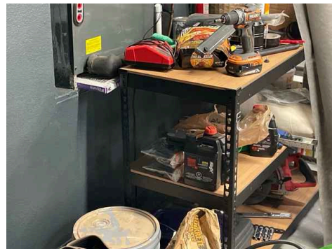
Shelf blocking filter removal
