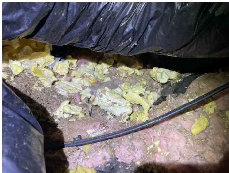
Insulation not removed from attic
