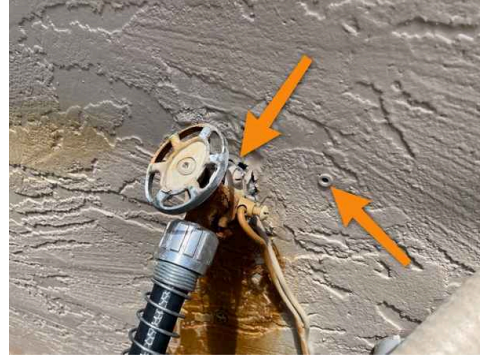
Left side by AC condenser
