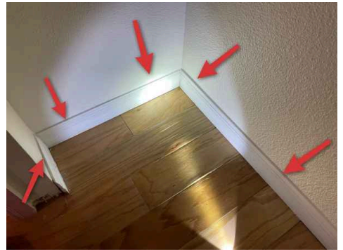
Baseboard separated from walls at right side of front left bedroom closet, closet shares wall with air handler
