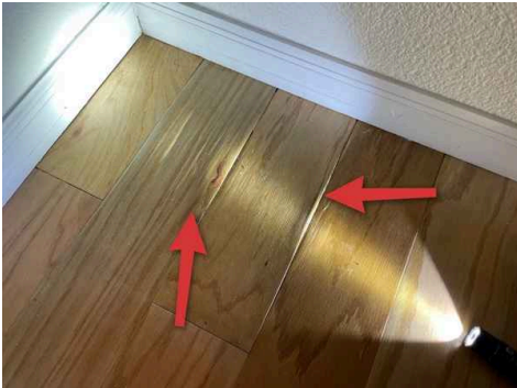
Water damaged flooring at front left bedroom closet, closet shares wall with air handler
