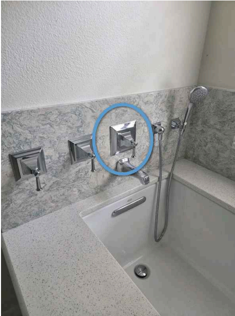
Master Bathroom, no cold water
