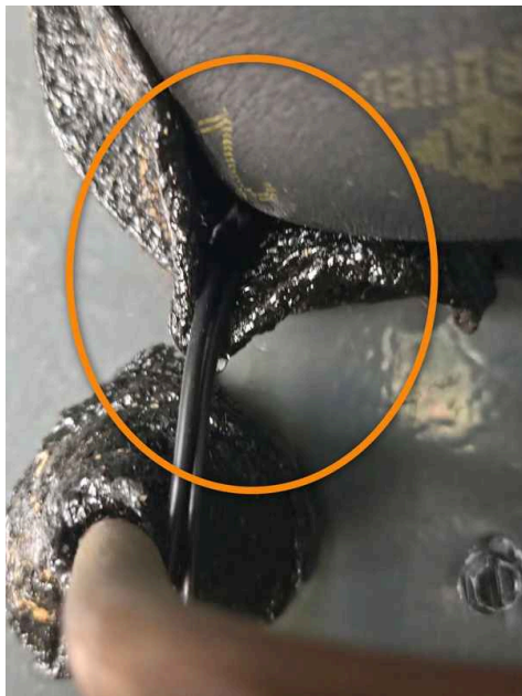
Unit in garage leaking
